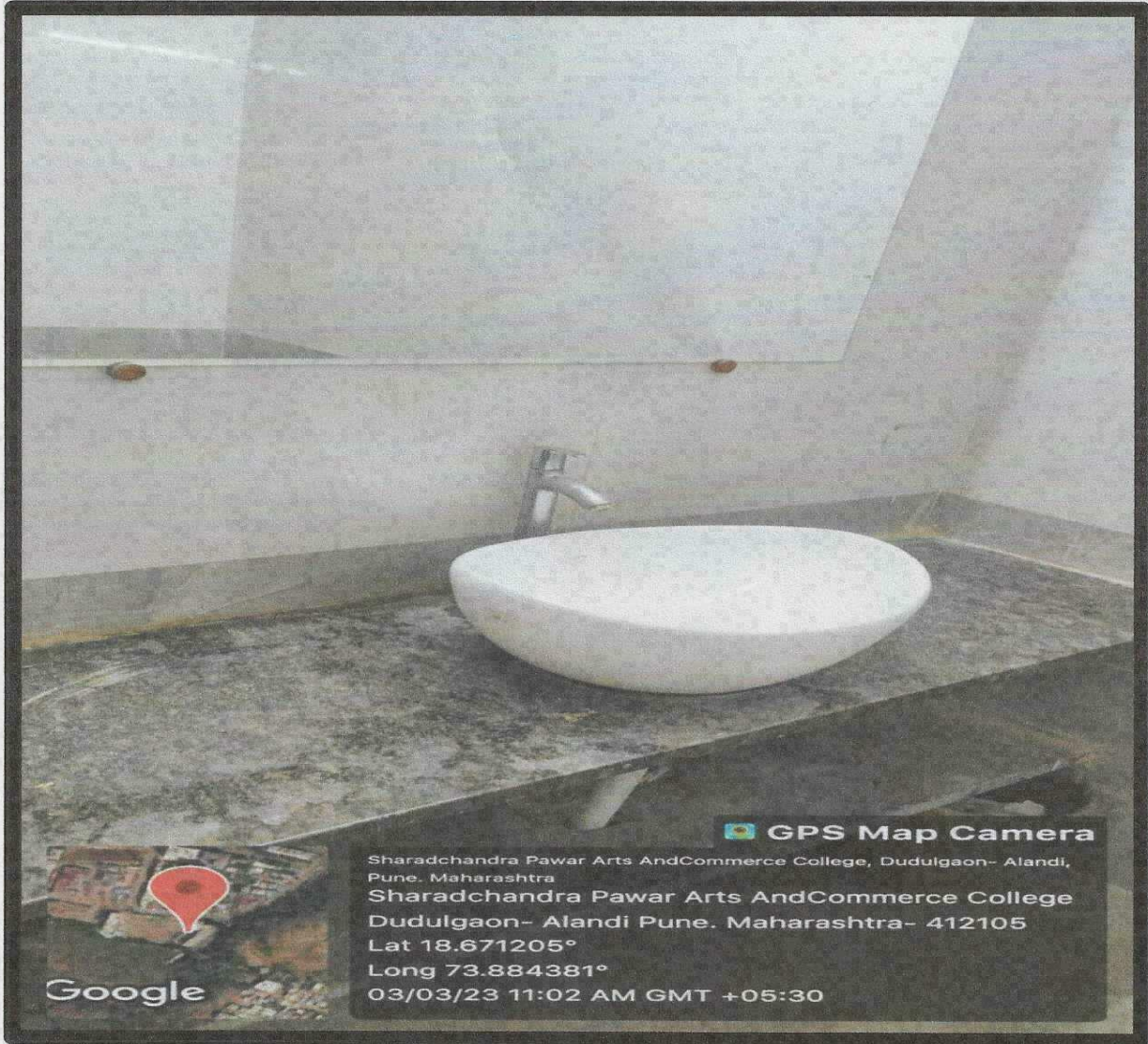
Basin of Physically Challenged Washroom
